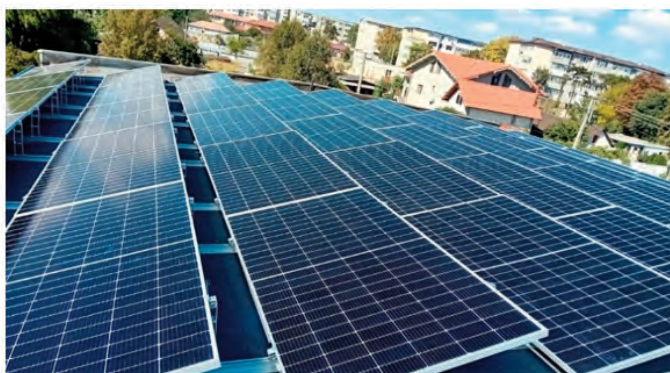
CEF SEAU Mangalia / Mangalia WWTP PV Power Plant
