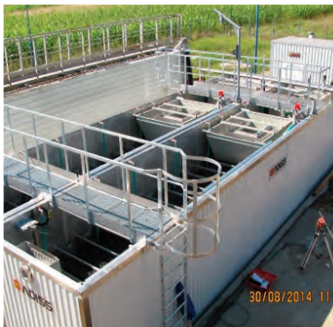
Fig. 8. SEAU Bradu - instalare module de epurare / Bradu WWTW - installation of treatment modules
