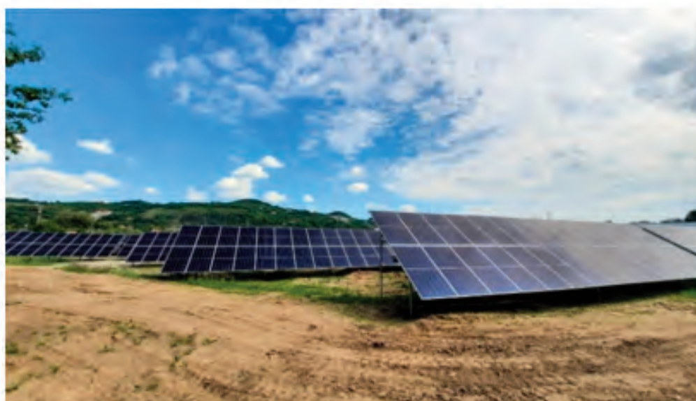
Fig. 14. Panouri fotovoltaice Sursa Florești / Photovoltaic panels Floresti Source
